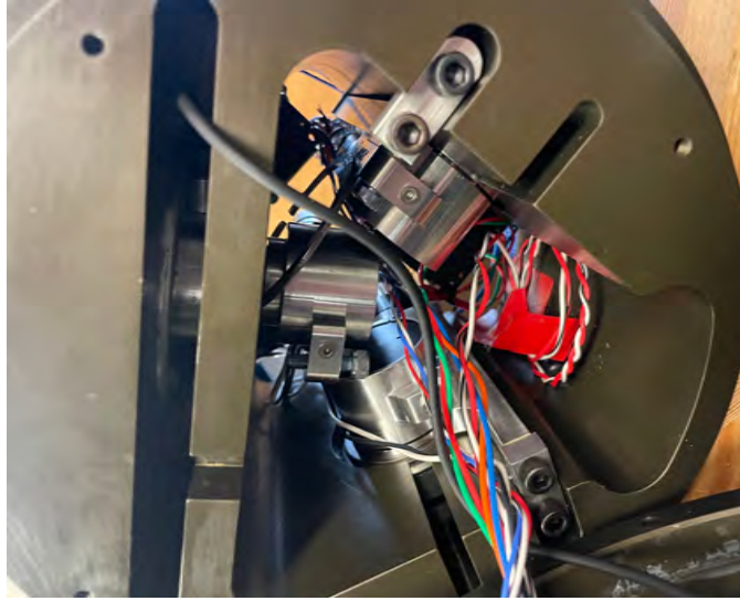
Figure 10: A view inside the rotor hub showing installed shaft seals, load cell, and gear boxes. The challenges with designing and installing these components ultimately determined the required diameter of the AFT.
