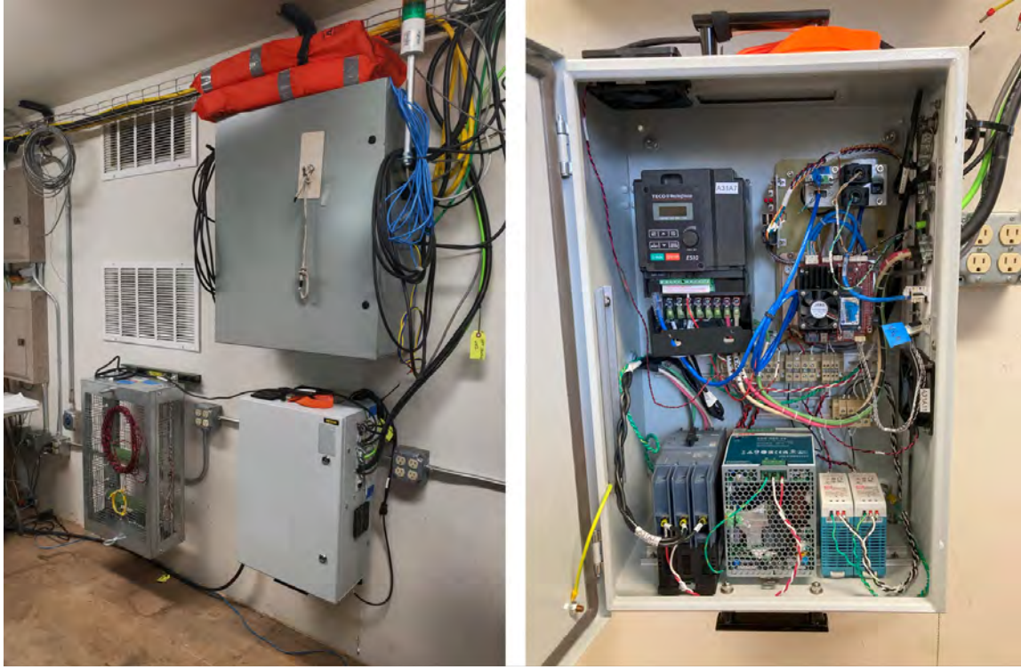
Figure 4: (left) The electronics enclosure and load dump installed in the lab on R/V Russell Davis Light . The AFT enclosure is the unit located lower on the wall. Cables exiting the electronics box are routed through the container walls to the gantry/frame where they are secured to AFT's support structures.
