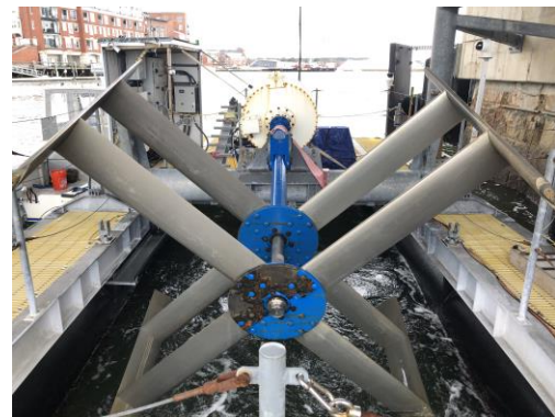
FIGURE 2: NEW ENERGY MODIFIED ENVIROGEN-025H CROSS-FLOW TURBINE INSTALLED ON UNH TURBINE DEPLOYMENT PLATFORM (SHOWN ROTATED OUT OF WATER).
