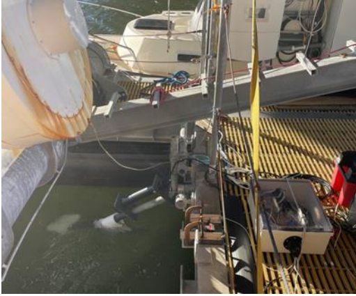
FIGURE 16: BENT ADV DEPLOYMENT PIPE (UPSTREAM) ON 12/8/22. PHOTO BY MICHAEL MONAHAN/ UNH.
