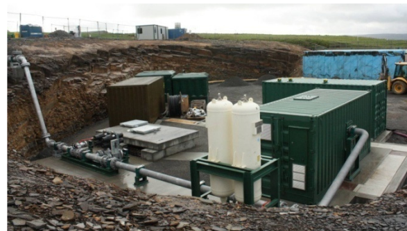
Figure 4: Oyster 1 onshore power station at EMEC
