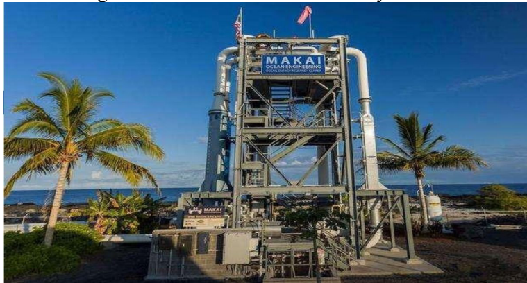
Figure 1. Traditional Ocean Thermal Energy Conversion System
