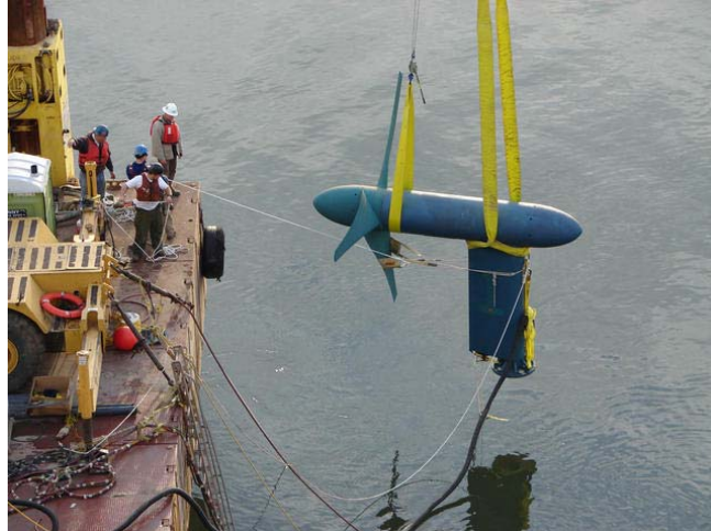
Figure 84 Verdant Power Turbine being lowered into the East River prior to mounting with a monopile
