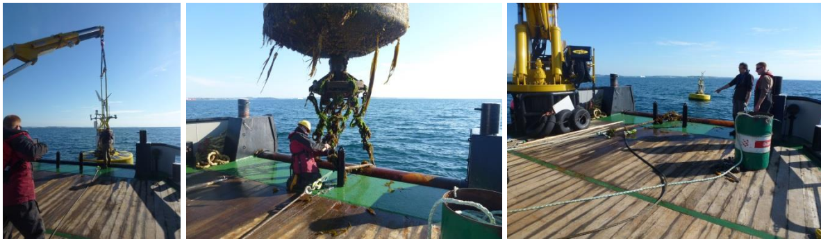
Figure 15: Example operation showing recovery of one SWMTF mooring rope using on-board crane and winch of the work boat
