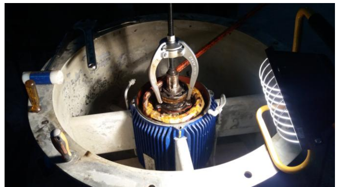
Figure 10: Greasing of roller bearings during scheduled maintenance work.
