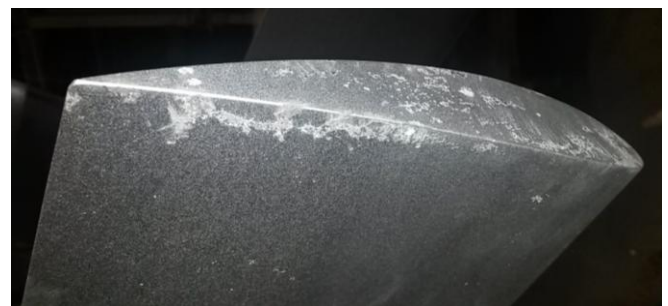
Figure 7: Salt accumulation on the surface of the Wells turbine blade.
