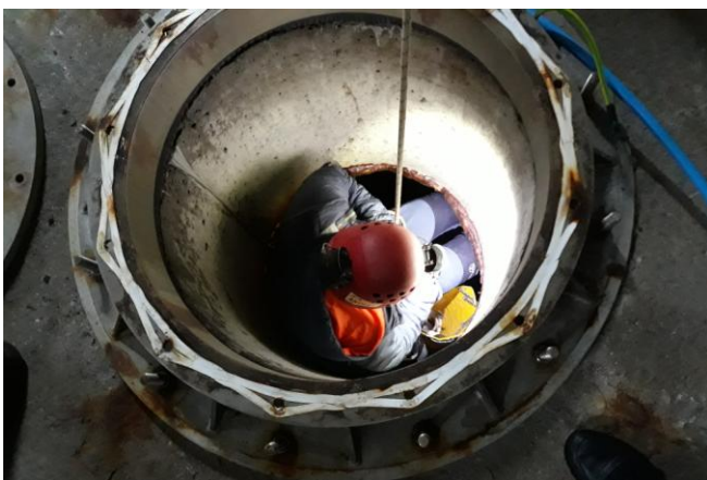
Figure 7: An operator accessing the chamber through the turbine orifice during sensor installation process
