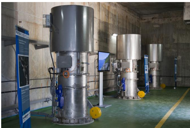
Figure 1: Turbo-generator modules installed in Mutriku Wave Power Plant
