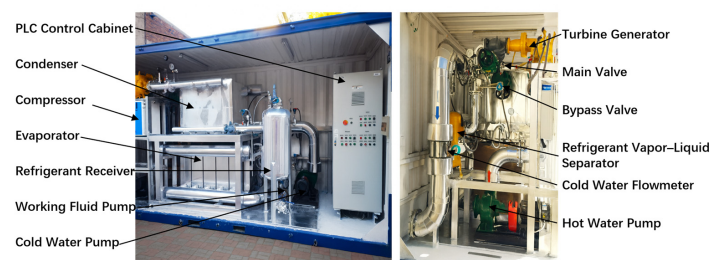
Figure 5. Containerized OTEC prototype system used for land-based and sea trials. The left image shows the complete integrated power module with its control cabinet, condenser, evaporator, and pumps, while the right image provides a detailed view of the turbine-generator and auxiliary subsystems.
