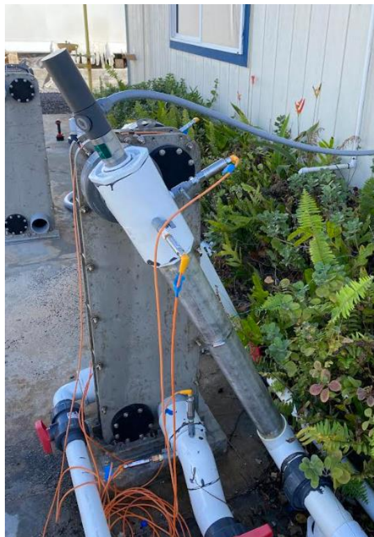
Figure 38. Zeta Rod installed in FL-1 slot.
