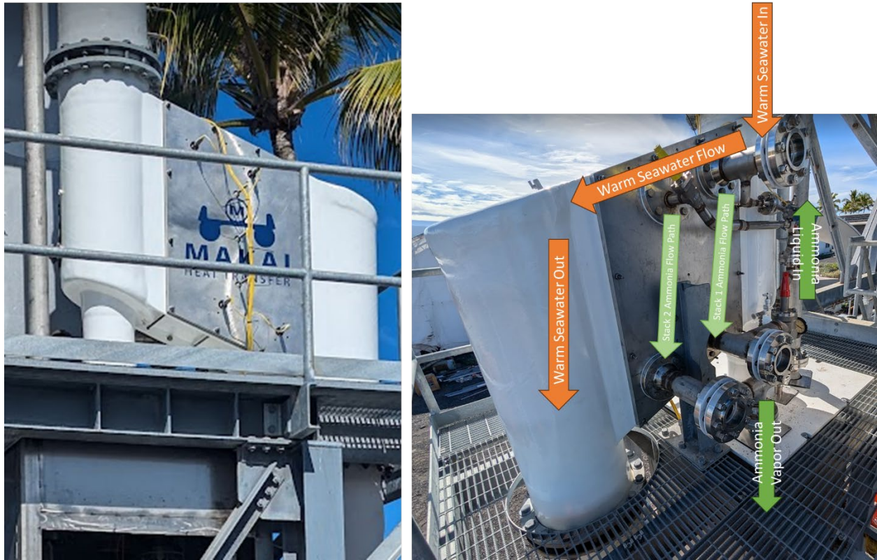
Figure 4. Evaporator installed in HX Tower
