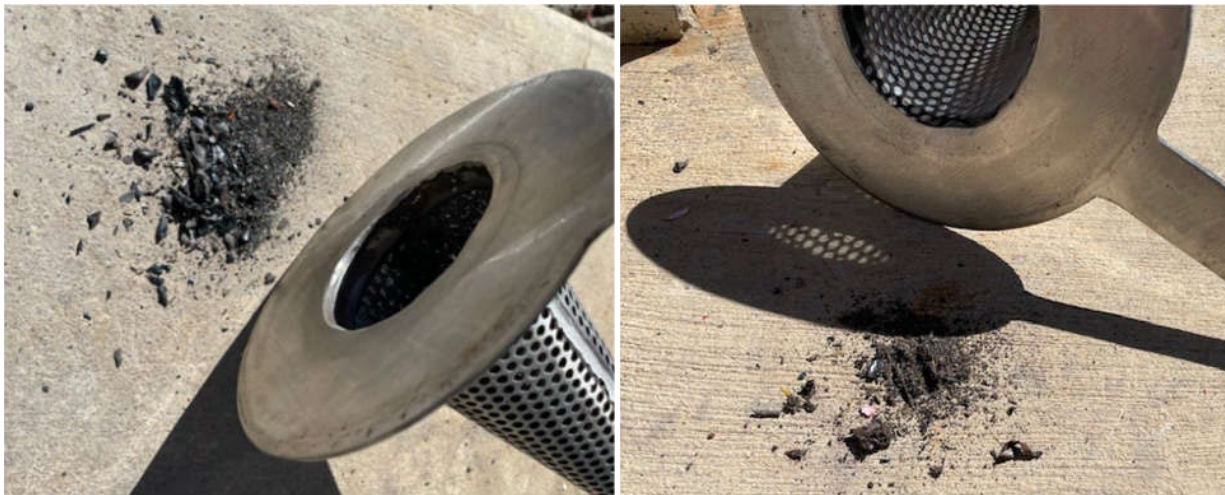
Figure 6. Debris in ammonia piping caught in strainer.
