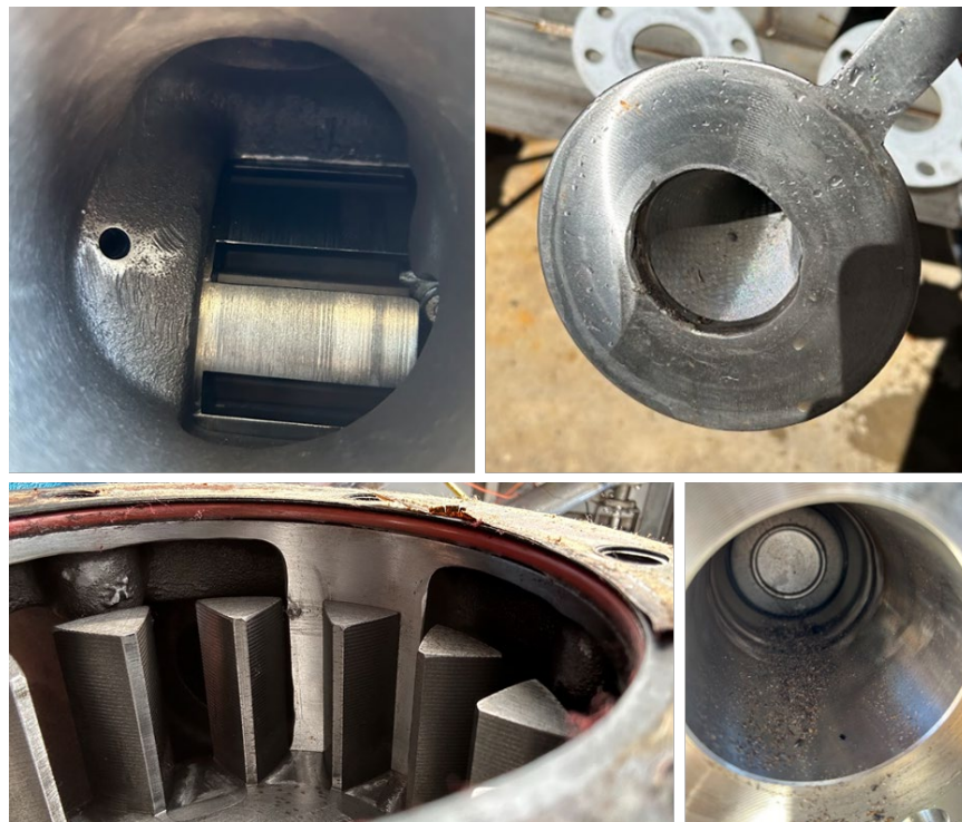
Figure 8. Feed pump damage.
