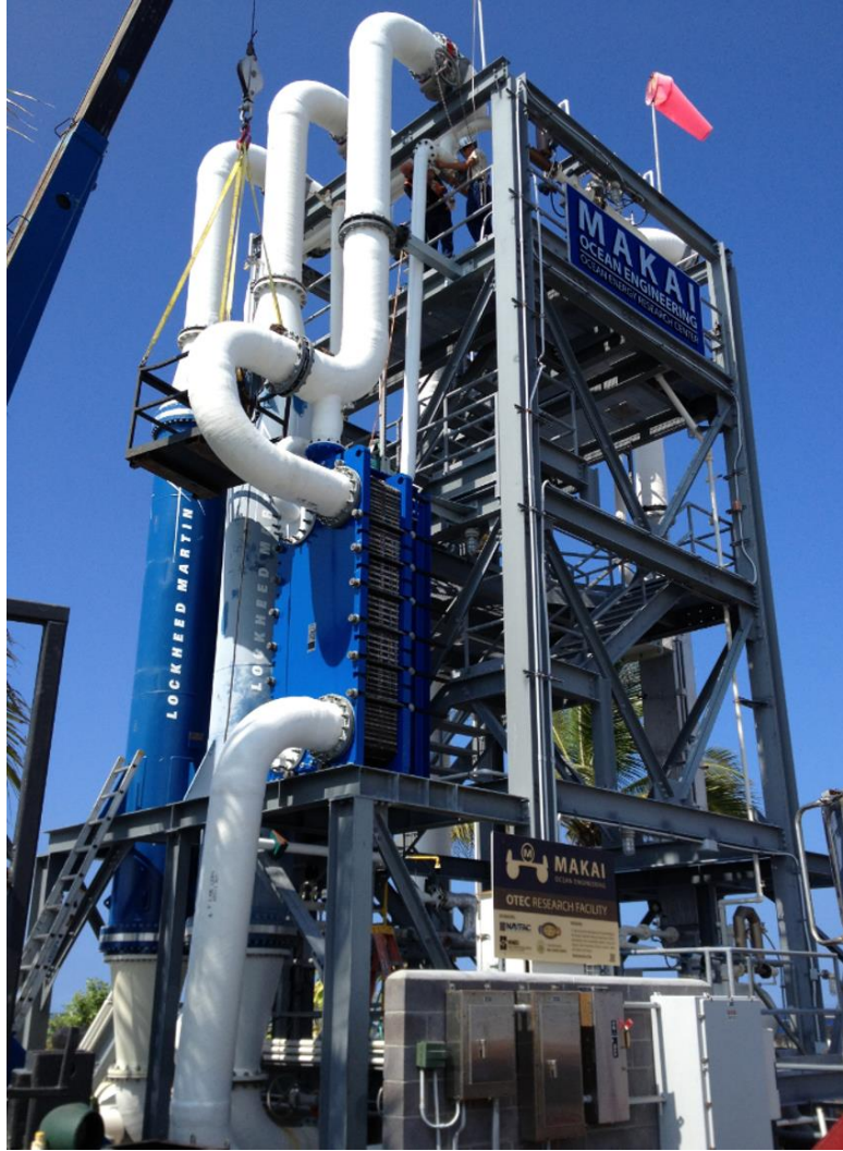
Figure 3-1. APV Titanium plate-frame heat exchanger installed on the OERC HX Performance Testing Facility.
