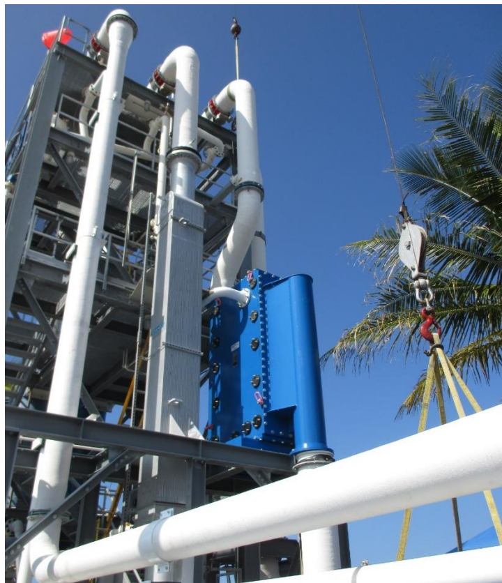
Figure 3-9. APV Cross Flow Heat Exchanger installed at the OERC HX Performance Testing Facility.
