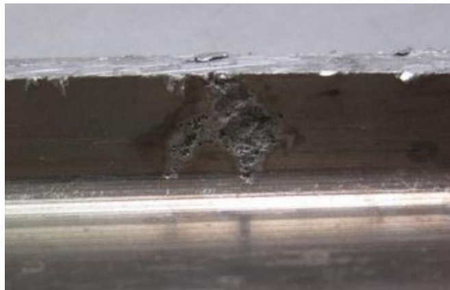
Figure 4-6. One of several large pits on LA83P samples in DSW. These pits are located along the sides of the sample and cannot be scanned by the profilometer.
