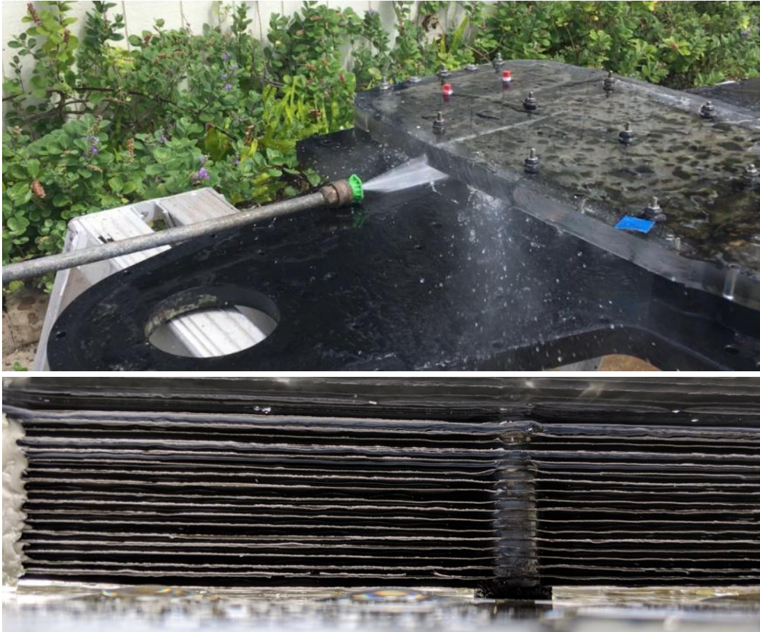
Figure 31. TFHX plates after water nozzle test.
