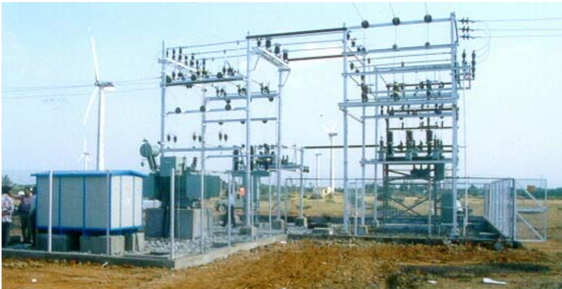
Figure 10-12 Fixed and Switched Capacitor Bank Supporting a 2.8-MW Wind Farm in India (Source: Crompton Greaves Ltd.)
