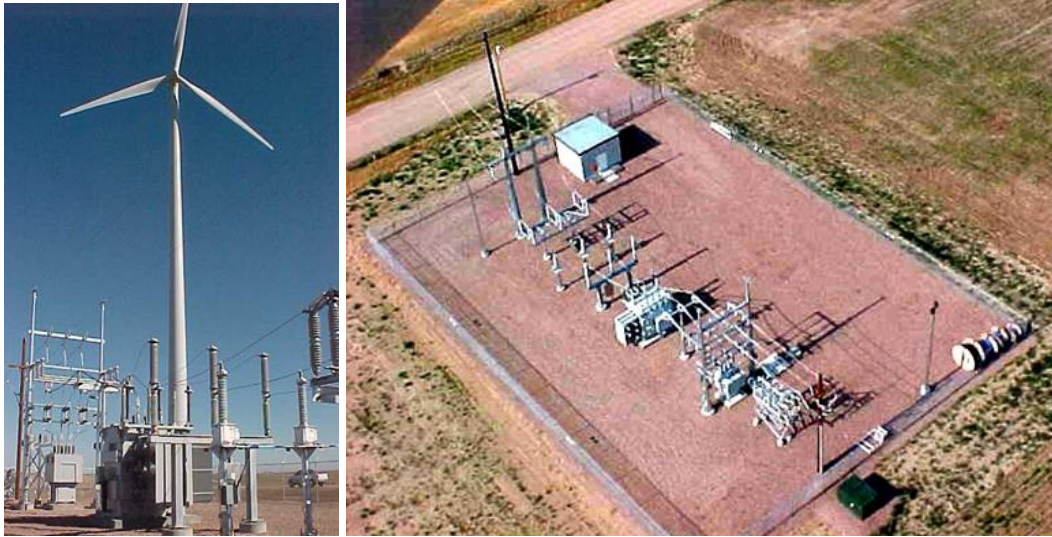
Figure 10-3 Grid Interface for Peetz Table 30-MW Wind Farm
