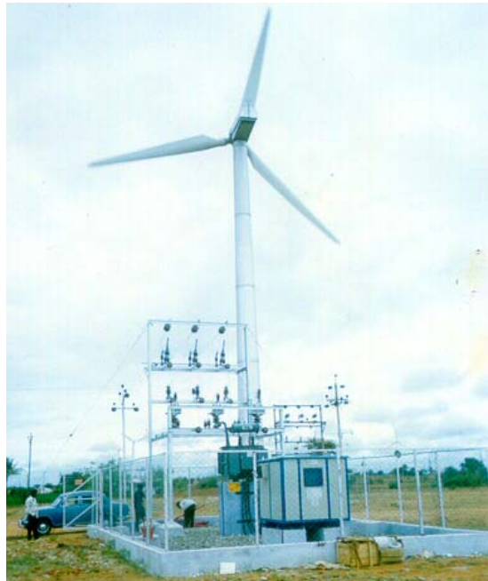
Figure 10-16 Distribution Static VAR Compensator (DSVC) at Wind Site in India (Source: Crompton Greaves Ltd.)
