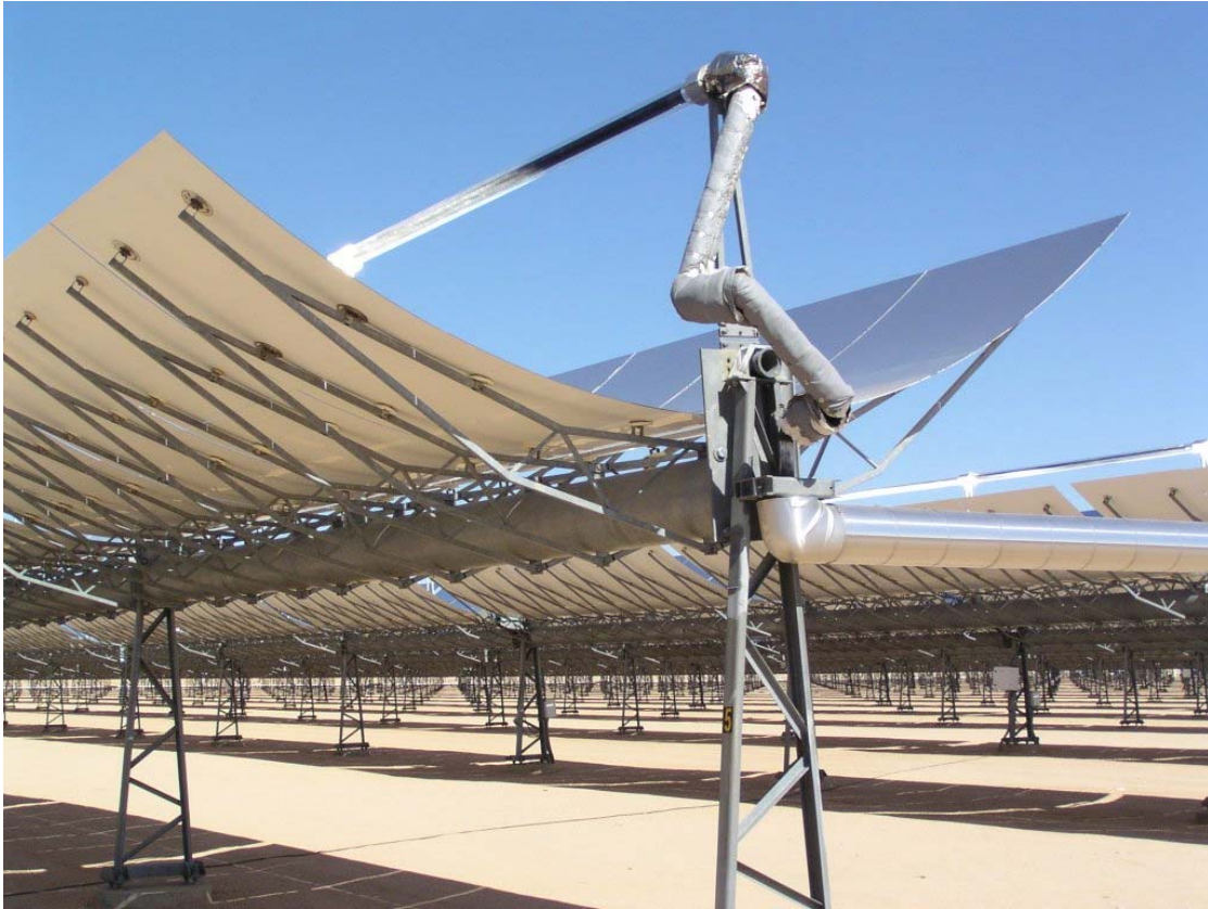
Figure 7-2 Solar Trough Collector Field at Kramer Junction, California. Note the receiver tube at the reflectors' focal point that transports heat-transfer fluid.
