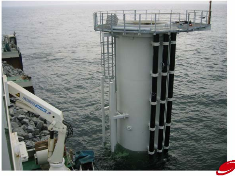
Figure 3-13 Monopile Steel Foundation and Transition Section for Wind Turbine at Horns Rev Offshore Wind Project (EUREC, Elsam, and Risoe National Laboratory [60])
