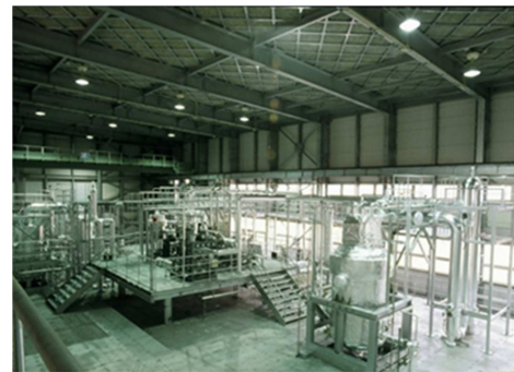
Figure 3: 30 kW OTEC and Desalination Room, Saga-Japan [IOES]
