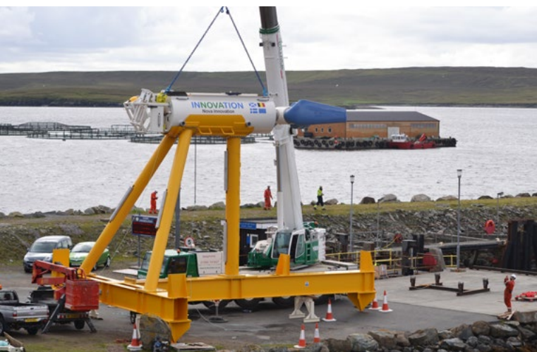
Nova Innovation M100 during assembly in Shetland Islands, Bluemull sound, UK Courtesy: Nova Innovation
