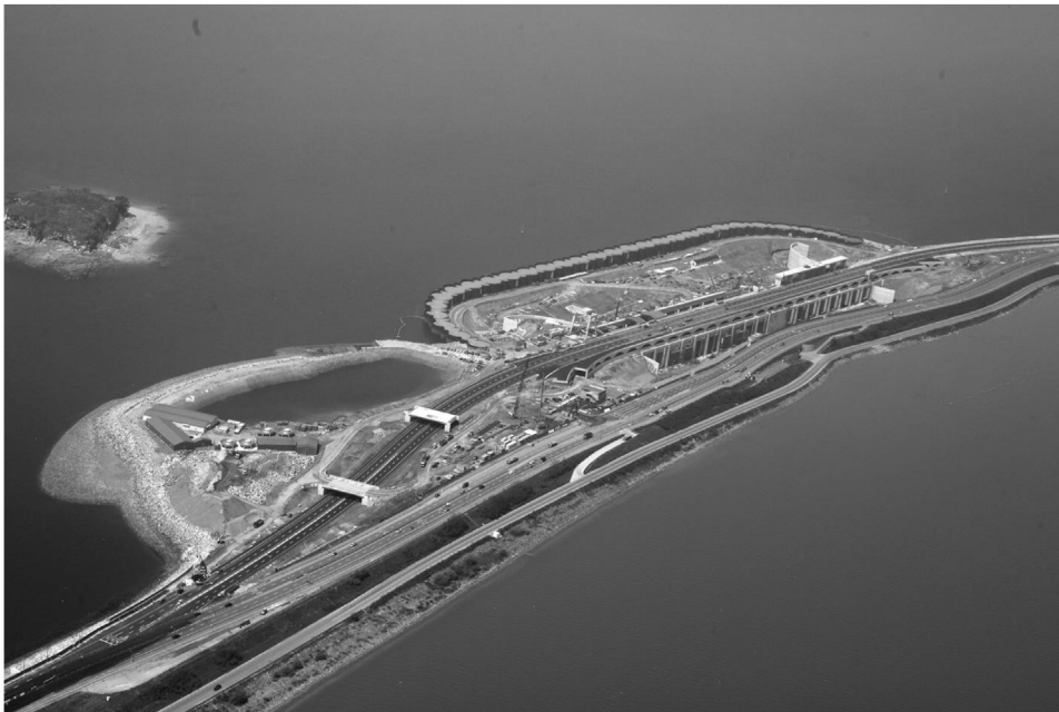
Fig. 16. Overview of the circular cell and arc cell temporary coffer dam construction site.
