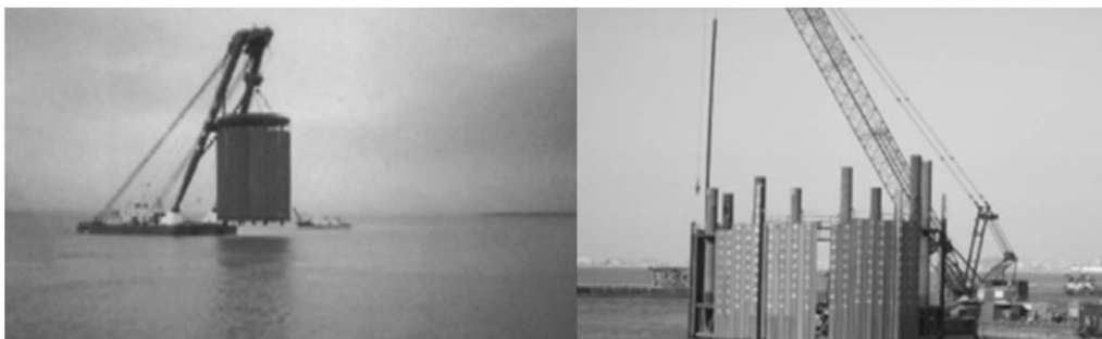
Fig. 14. Circular cell on land construction and marine transportation (left), on-site installation (right).
