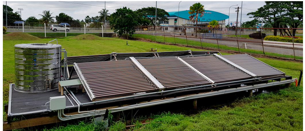
Figure 1. A photograph of the evacuated-tube solar water-heating system.
