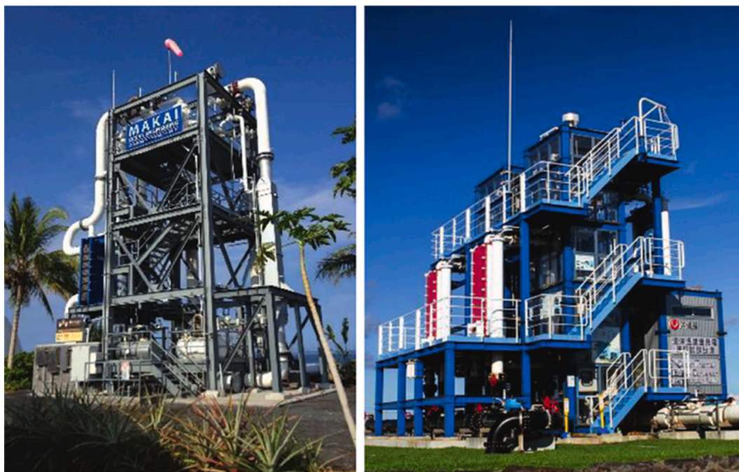
Fig. 9. Operating OTEC installations in Hawaii (left) and Okinawa (right) [59].
