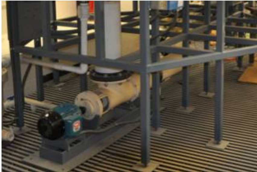
Figure 12. Water Tunnel Two pump.
