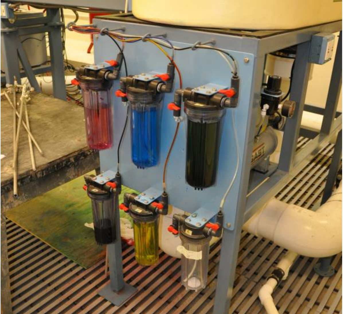
Figure 14. Dye injection containers in front of the air compressor.
