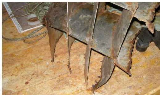
(b) Failed, pictured 10/2009
