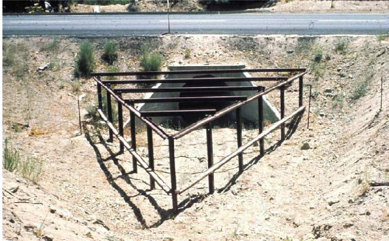
Figure 7: Debris deflector placed upstream of culvert opening (Lagasse et al., 2010)
