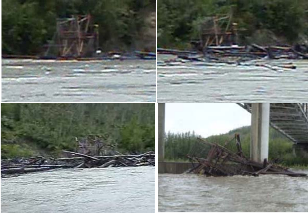
Figure 3: Large entangled debris event impacting (upper left) and carrying off (upper right and lower left) a fish wheel on the Tanana River near Nenana, Alaska, and depositing it against a bridge pier (lower right) (courtesy of Stephen Lord)
