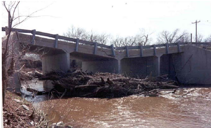
Figure 4: Debris accumulation on bridge piers and the resulting failure (Lagasse et al., 2010)
