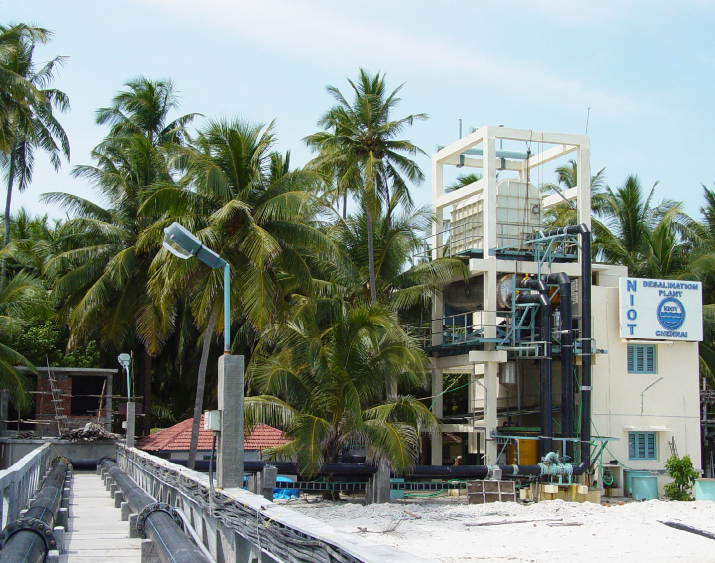
Water desalination plant at Kavaratti Island Courtesy: NIOT
