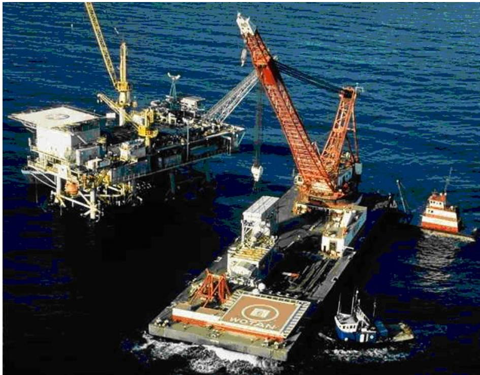
Figure 21 - Manson Construction 600 ton Derrick Barge WOTAN operating offshore In heavy currents these barges use a mooring spread that allows them to keep on station and accurately reposition themselves continuously using hydraulic winches controlled by the operator.
