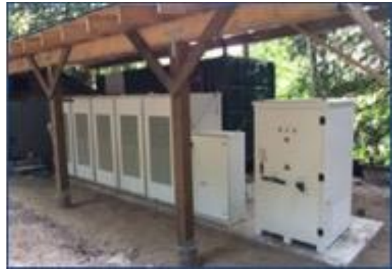
Microgrid & Energy Storage
